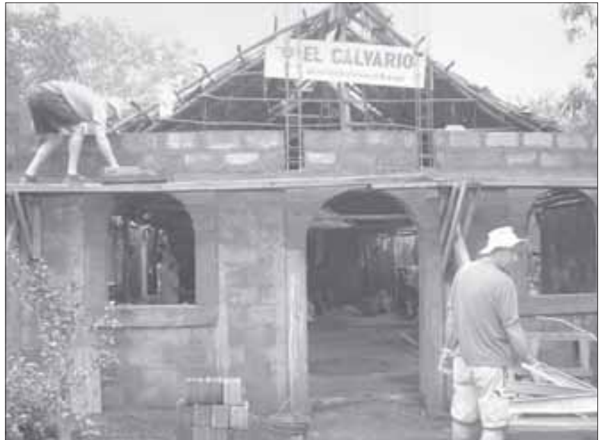
New Roof and walls made El Calvario a safer place for worship and Christian education
